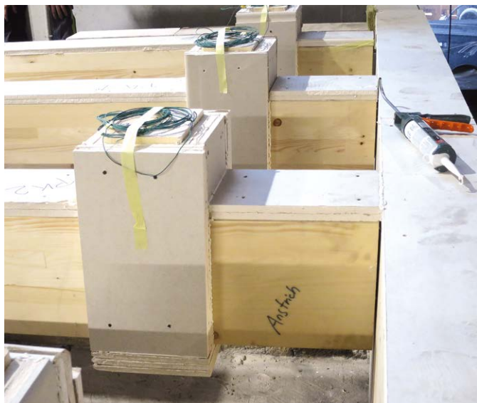
^ Application of the fire protection coating “Fire Shield” on the secondary beam
