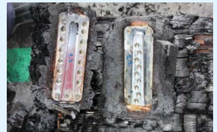
^ SHERPA system connectors after the fire test of 120 minutes.
